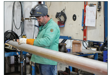
Pipefitter Mike Laesch checks to make sure the pipe he is about to weld is level.
