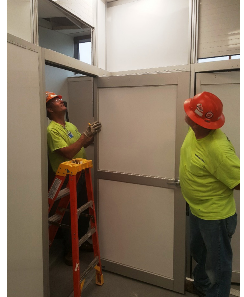
Jim Babkiewicz (left), RLI carpenter general foreman, and Rick Turner, RLI superintendent, working on ICRA panels at the Mercy Perrysburg project.
