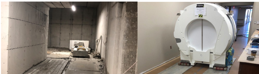
L-R: Concrete demo to expand the vault entrance and the Gamma Knife unloaded onto aluminum plates.
