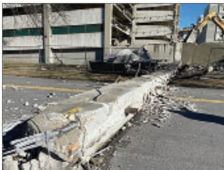
There is always the possibility of an uncontrolled collapse during demolition.
