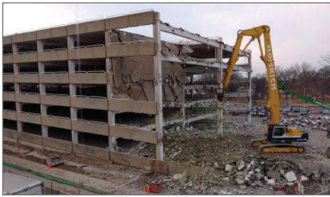
Communication is the primary key to success during a demolition such as the one at St. Vincent Mercy Medical Center.
